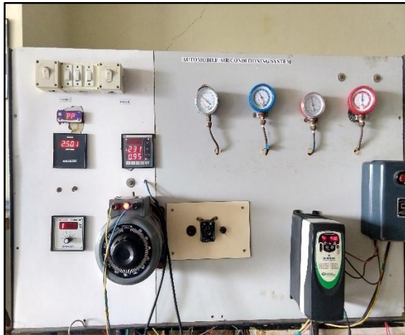
Fig. System Controls
